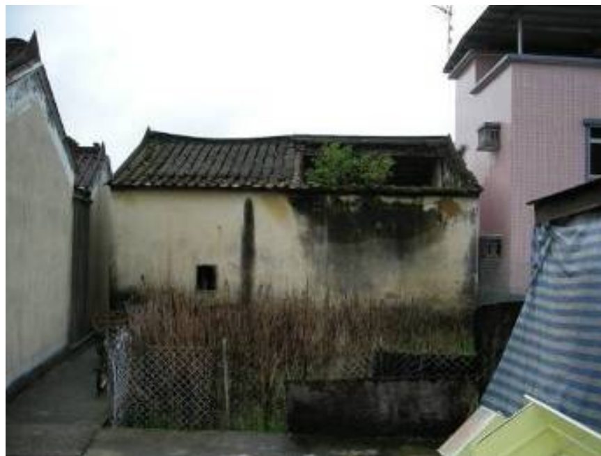
Back view (collapsed roof)
